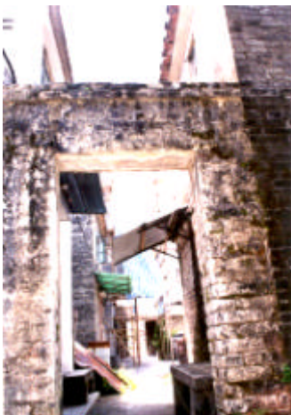
Old Walled Village Structures Are Vulnerable to Deterioration
